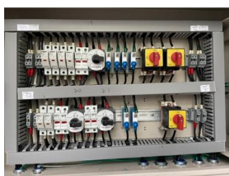
Switches of Solar Panel of MG2 and MG3
