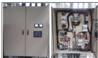
Switches of Interconnected System
